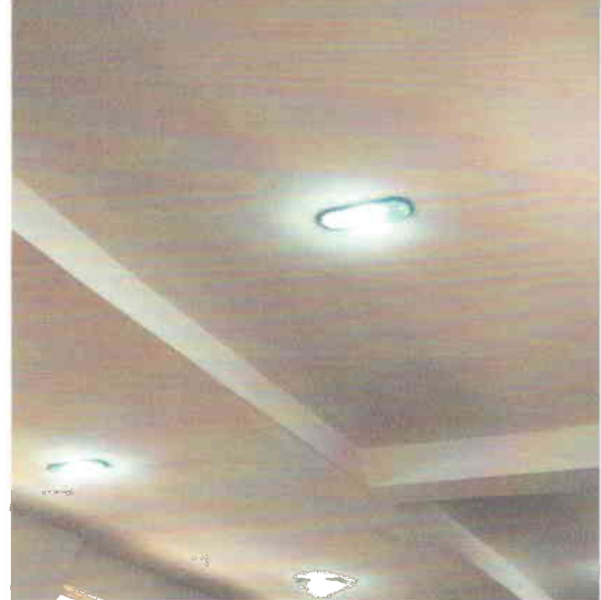
LED BULBS IN KAMARAJAR BUILDING
