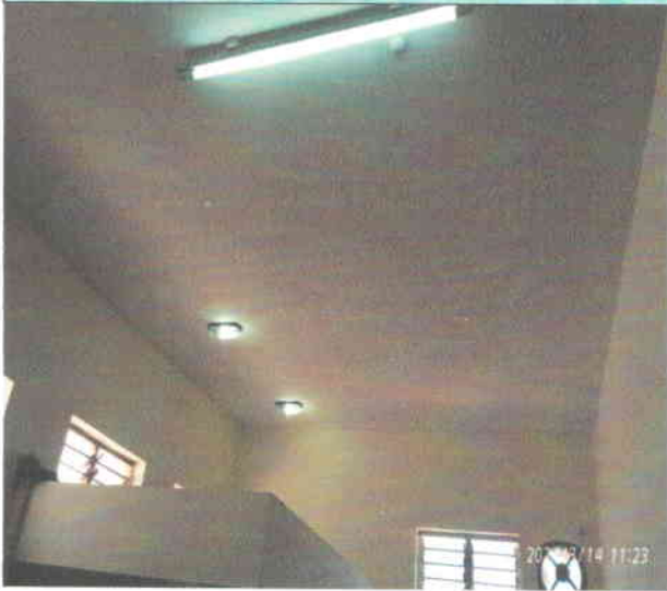
LED BULBS IN MAIN BUILDING
